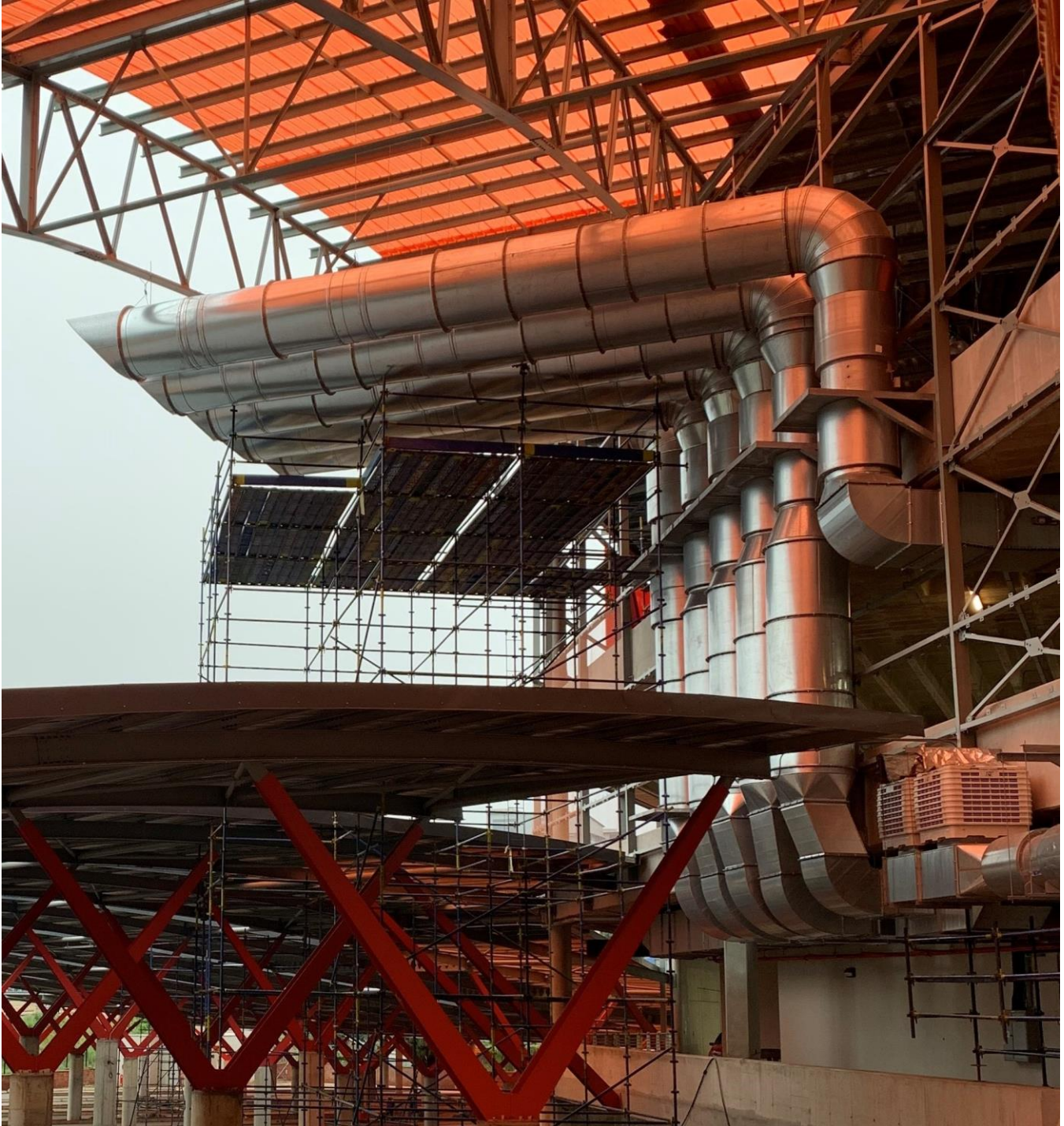
Photo of Smoke Exhaust system at the Kazerne International transportation hub Johannesburg.
